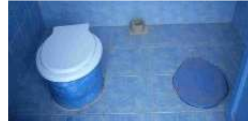
Poor ventilation design
